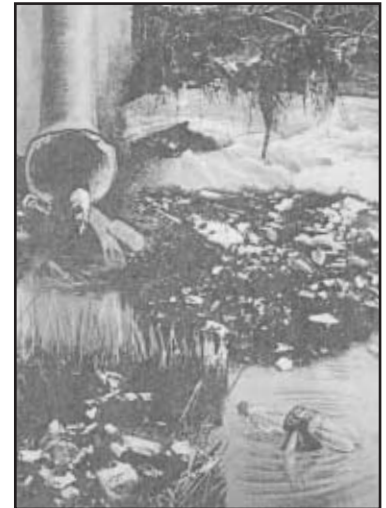
Sewerpipe Brian Bainbridge
